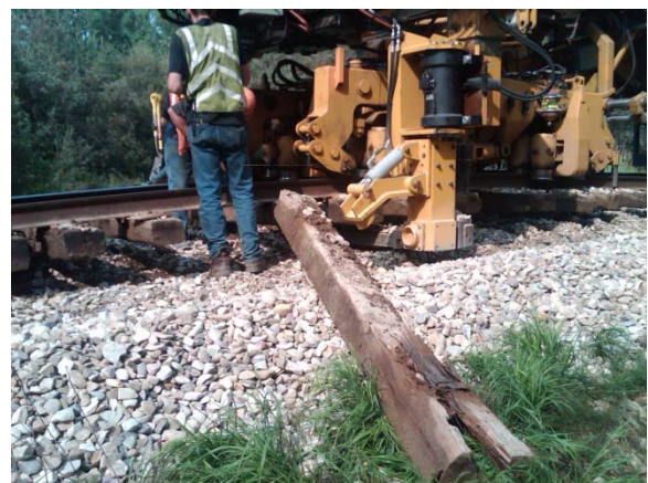
(Fig 5 - Tie failure discovered while lifting on ANY)
